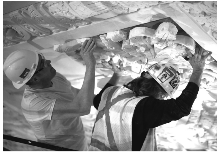
During the renovation, workers put a piece of decorative art in place in the new auditorium of Northrop.
