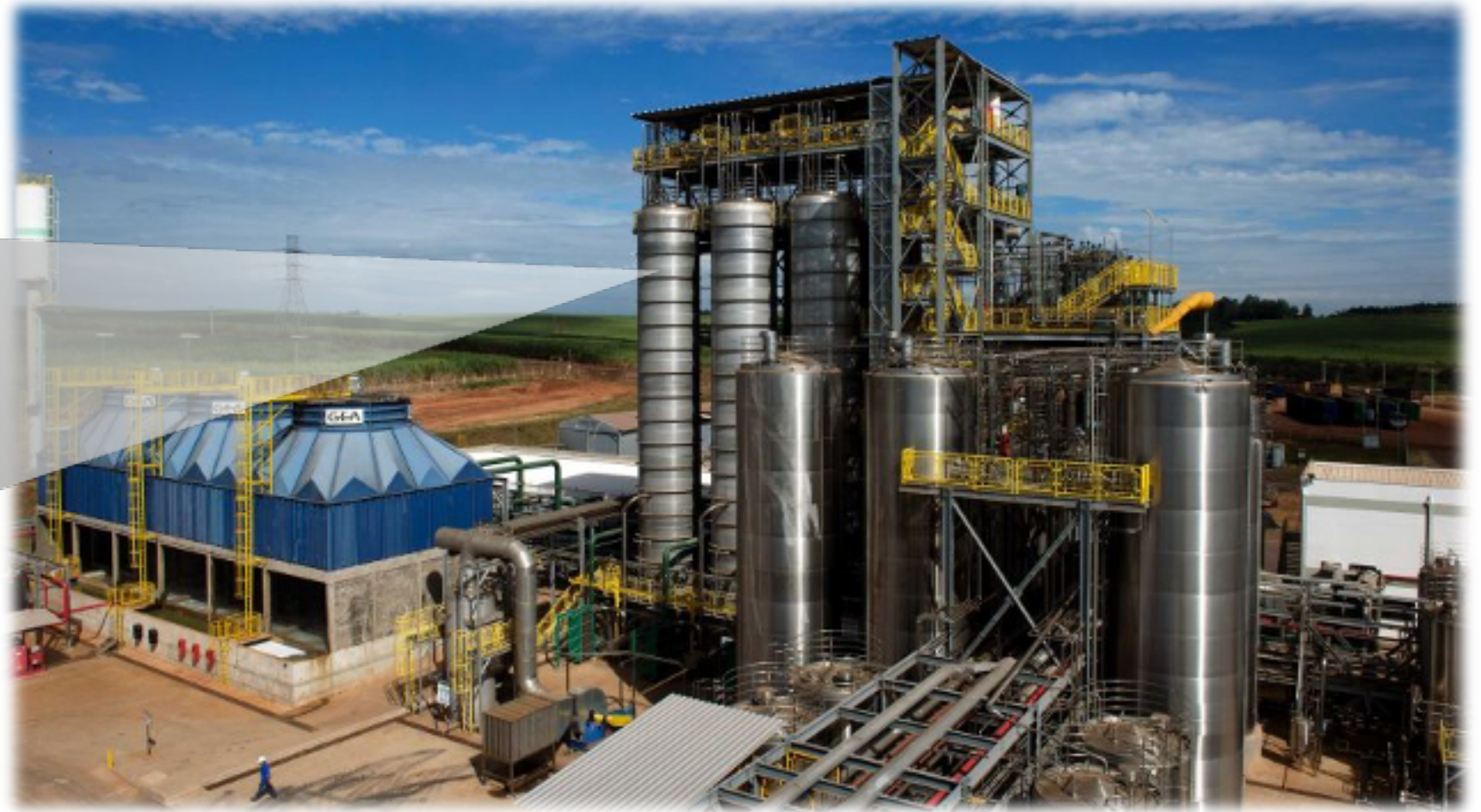
200,000 L Fermentation tanks at Amyris' Brazil Production Facility
